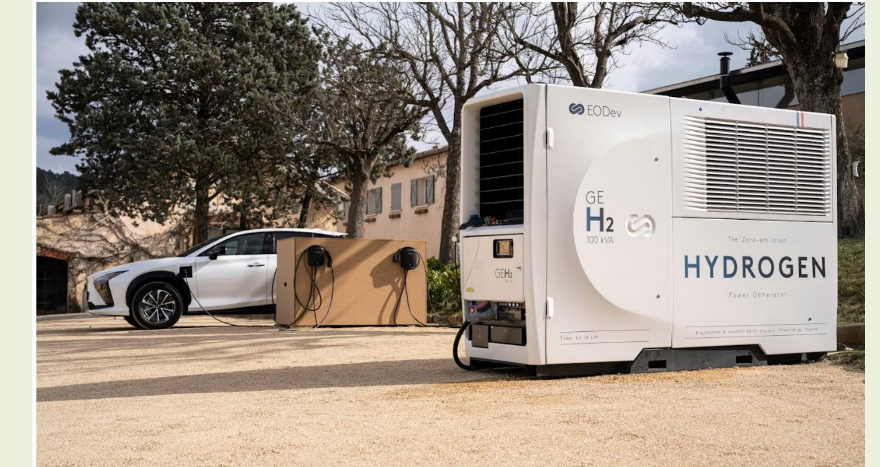
Hydrogen burning electricity generator
